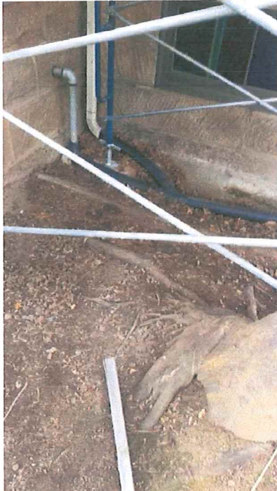
Tree 2 roots going under foundation.
